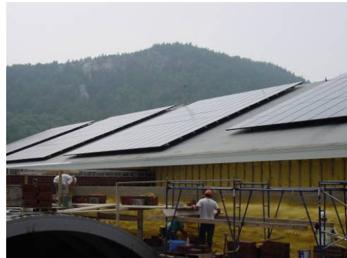
A 56 kW solar photovoltaic array was installed on this middle school's south-facing roof. The array will supply 9.9% of the school's as-designed energy needs.
