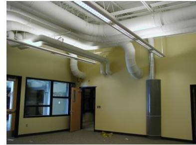
Displacement ventilation is being used in this high school as an efficient means of providing ventilation and dehumidification for interior spaces. The supply air will be delivered through floor or wall-mounted diffusers (see gray diffuser on right wall in picture), designed to deliver air at low velocity. Supply air will typically be 100% outside air.
