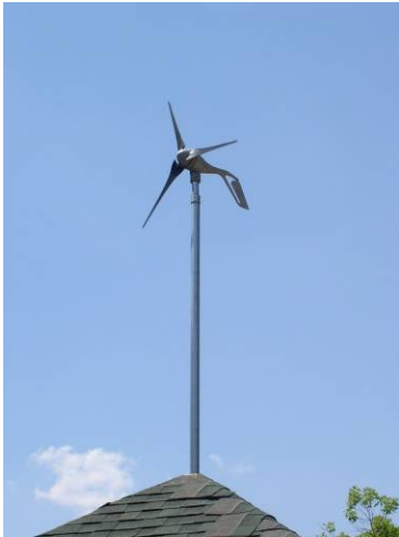
A small 400 Watt wind turbine was installed on the roof of this school's garden shed for demonstration and instructional purposes.
