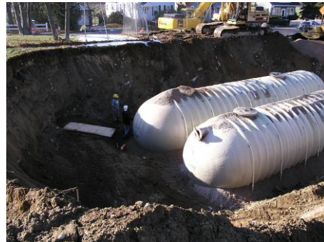
Two 25,000 gallon tanks were installed underground at this middle school. The tanks will store rainwater collected from the school roof. The rainwater catchment system was sized so that it can provide 100% of the water needed for sewage conveyance for the whole building and 100% of water needed to irrigate a small ball field on the site. No potable water will be used for irrigation or toilet flushing.
