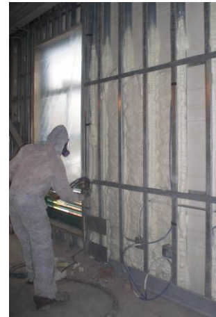
Spray foam insulation was used in this child center to create a tighter building envelope that will save energy and money.
