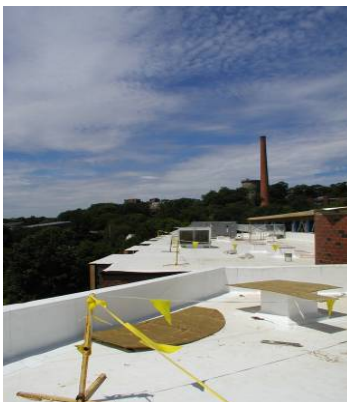
A white roof was installed on this elementary school to reduce heat island effect.
