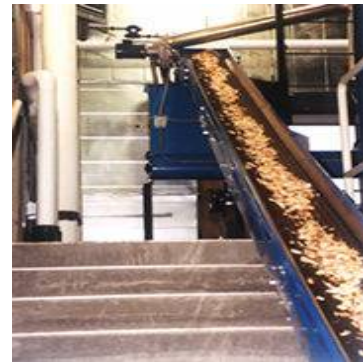
Conveyor belt for a biomass fired heating system.
