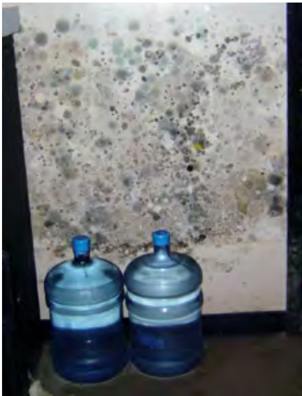
Mold growth on wall board.
