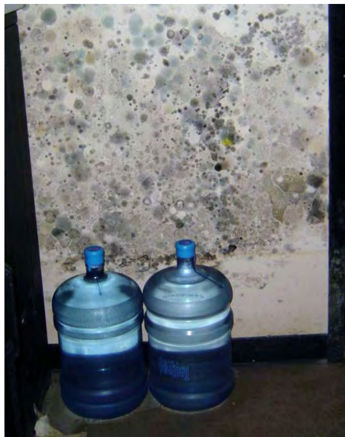
Mold growth on wall board.
