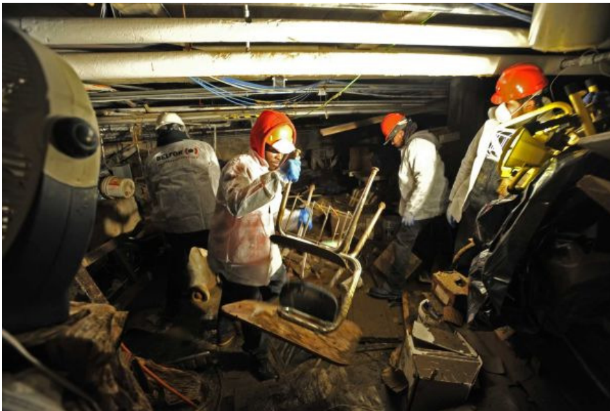
David Pokress | A recovery crew removes desks and chairs that were damaged during Sandy at East Rockaway Junior-Senior High School. (Nov. 8, 2012)
