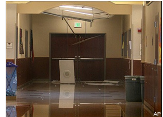
A broken ceiling piece hanging above a hallway after a 2,500 square foot section of roof at Capital High School in Olympia, WA collapsed in 2008. Olympia Assistant Fire Chief Greg Wright said the roof appears to have caved in due to the weight of snow, ice and water on top of the building. (AP Photo/The Olympian, Steve Bloom)
