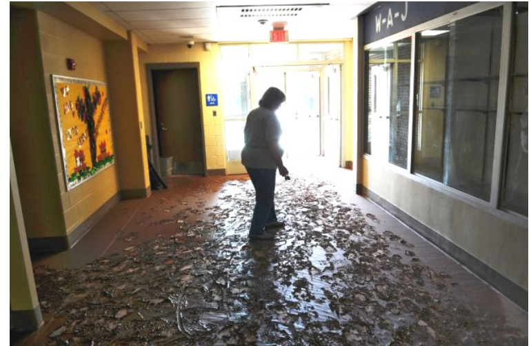
Mud coats the floors of the Windham Ashland Jewett Central School, damaged as a result of Tropical Storm Irene, on Wednesday Aug. 31, 2011, in Windham, NY. Michelle Mattice, treasurer of the school district, walks through the hall. (Philip Kamrass / Times Union)
