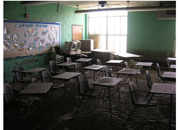
A school damaged by Hurricane Katrina. (Flickr, Paul Baker)
