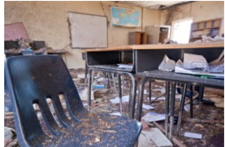
Tornado damaged classroom in the Tower Elementary school in Moore, Oklahoma. An F5 tornado struck the area on May 20th, 2013 causing widespread destruction. (Andrea Booher/FEMA)
